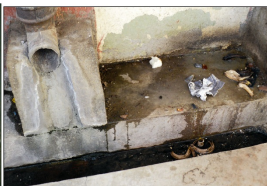
Disposal of liquid waste in municipal sewer system (Irvin Hospital)
